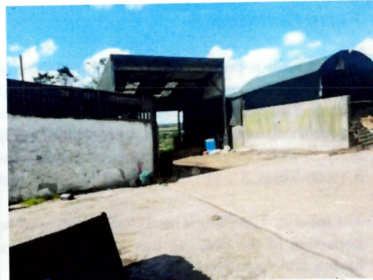
Plate 4-26 Exposed galvanised metal shed.
