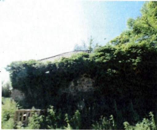
Plate 4-13 Dense ivy cover at rear.
